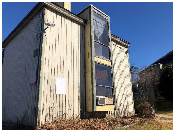
Building Rear Showing Needed Repairs
