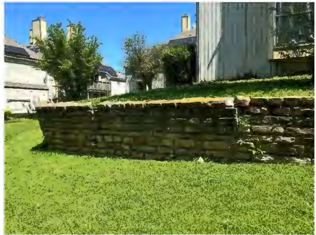
Cracked Retaining Wall
